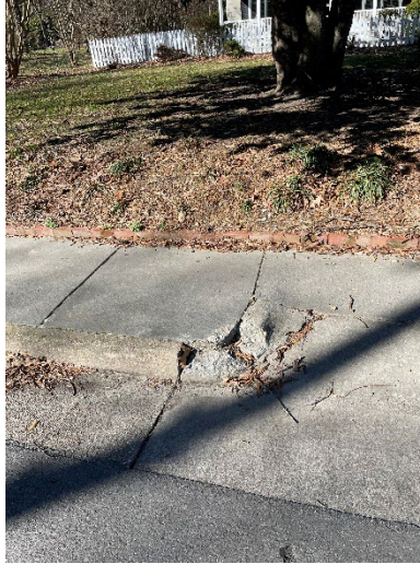
Item 10 – Deterioration of curb corner, 140 Steamboat Road
