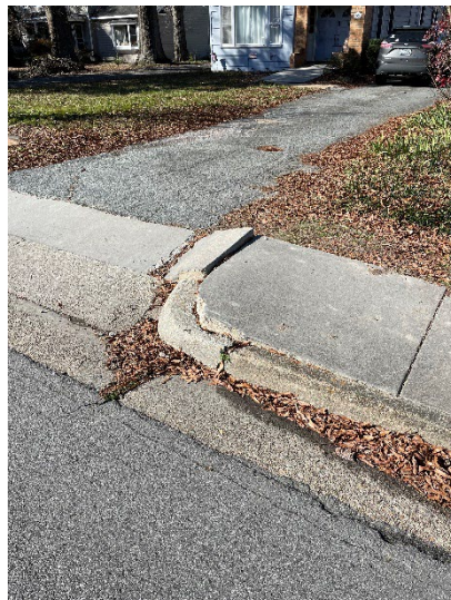
Item 12 – Major sidewalk and curb heave at 60 Steamboat Road
