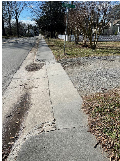
Item 11 – Both curb corners deteriorated at entrance of Bussels Lane at the next to 116 Steamboat Road
